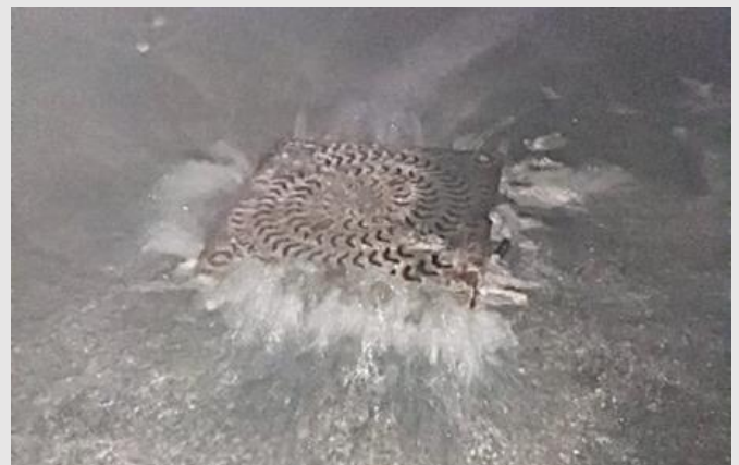
Overflowing Drain, Bosham High Street 16 th November 2022
